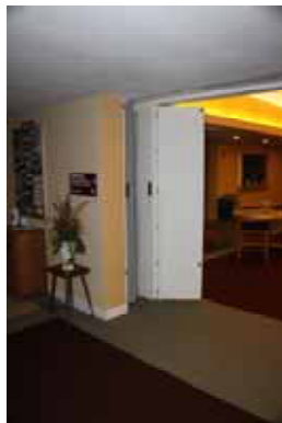
Wall panel open
