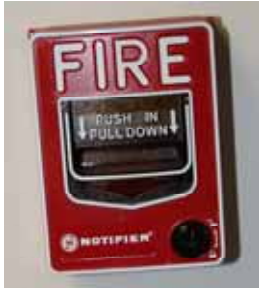
Alarm pull station
