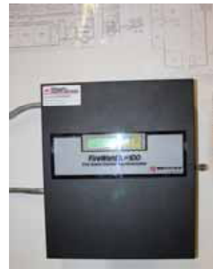
Control panel in maintenance room 117
