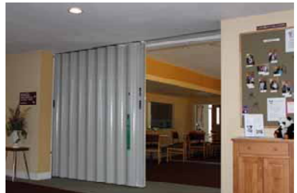
Fire door closing
